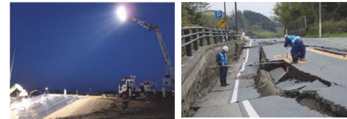
Emergency construction assisted by lighting car Investigation of road damage area (April, 2016 Kumamoto Earthquake)
